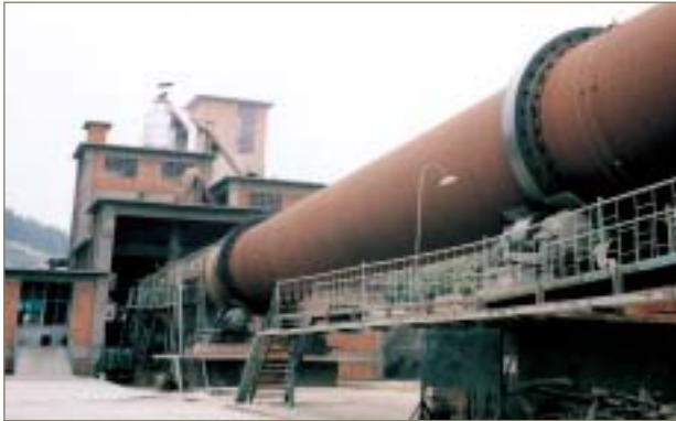
A rotary kiln of the cement plant in Kaili, Guizhou
